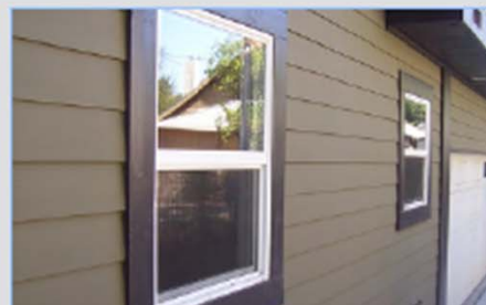
AVOID. The white window color is inconsistent with the color of the surrounding trim and cladding. White trim and perhaps a different color cladding material would result in a more consistent color palette.
