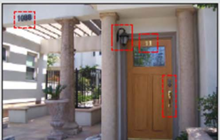
AVOID. Lamps, address signs, and columns are inconsistent in style and finish.
