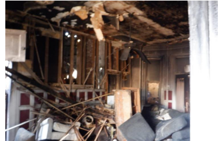
First story interior damages.
