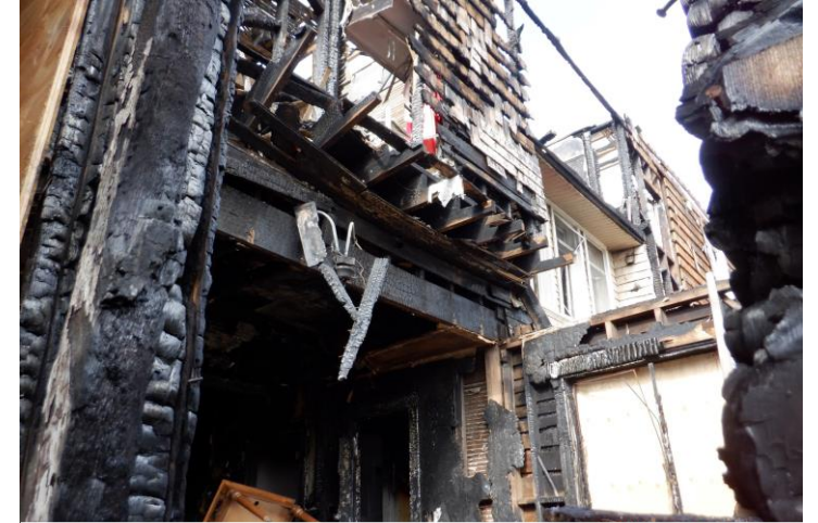
Fire-damaged exterior and interior structure.
