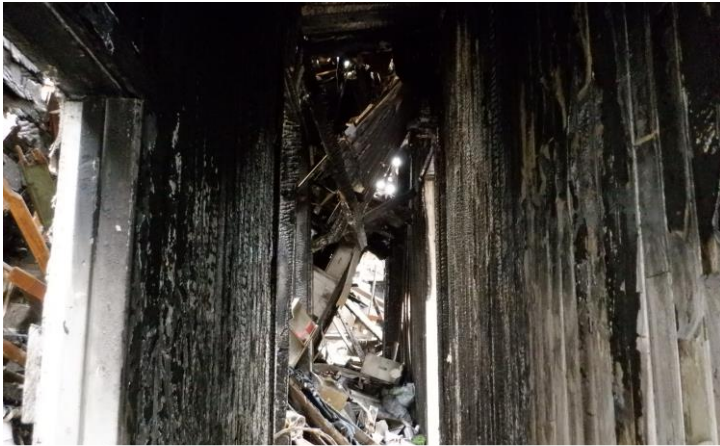
First story interior structural, fire, water and smoke damage.
