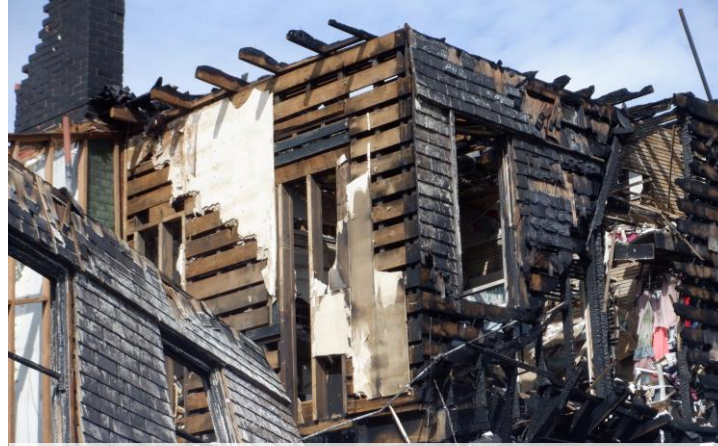
View of east second story exterior and interior walls, as viewed from neighboring east property.
