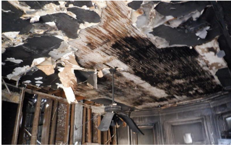
Ceiling of first-story dining room. Fire, smoke and water damage.
