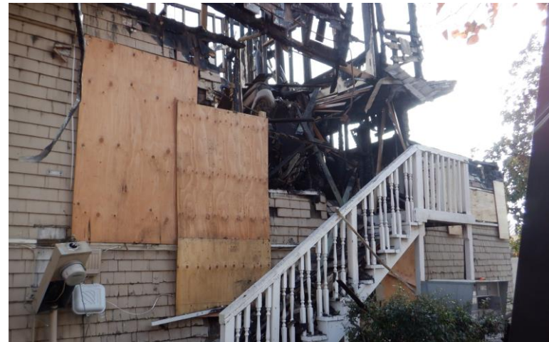
Remnant of SW second story exterior wall framing supported on door on stairs, warping under load.
