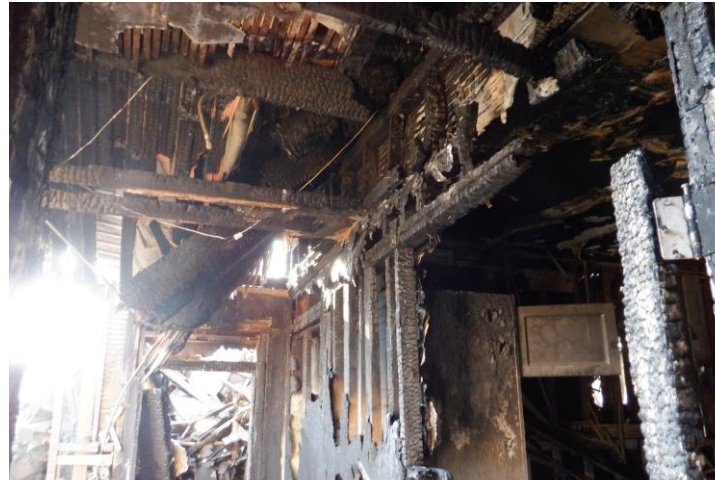
First story interior damages.
