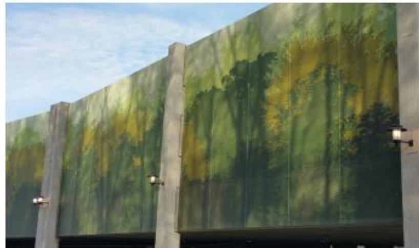
Crocker Park Parking Garage, Westlake, OH • Tensile Mesh Facade, Custom Printed with Tree Pattern Image
