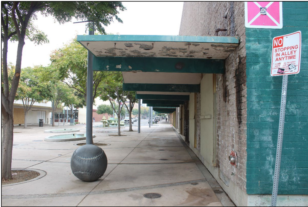
Figure 10. Detail of the cantilevered concrete canopy on the north façade of the building, facing northeast (Stantec, 2025).
