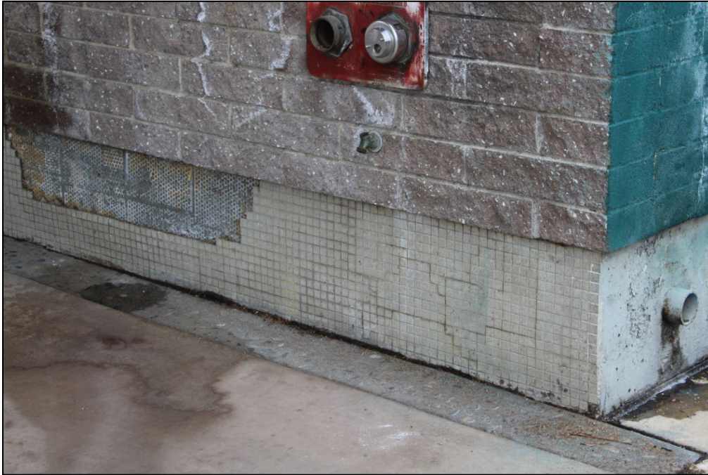
Figure 10. Detail of the cladding materials at the west corner of 887 Fulton Street, facing east (Stantec, 2025).
