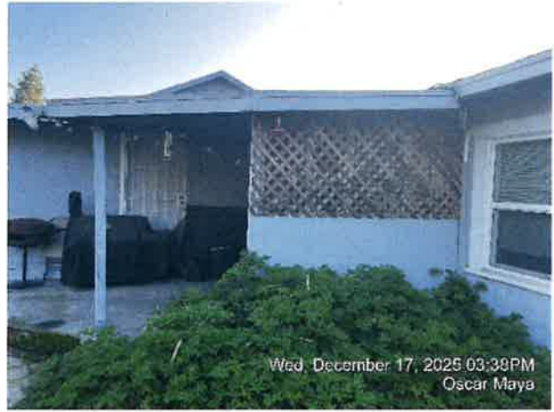
Date: 12/17/2025 03:38:59 PM Violation 1: Patio without permits.
