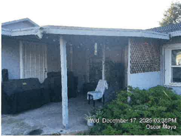
Date: 12/17/2025 03:38:27 PM Violation 1: Patio without permits.
