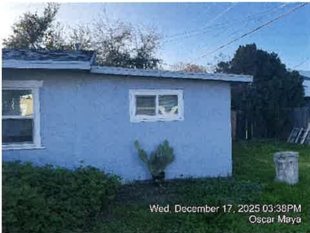
Date: 12/17/2025 03:38:31 PM Violation 2: Enclosed patio without permits.
