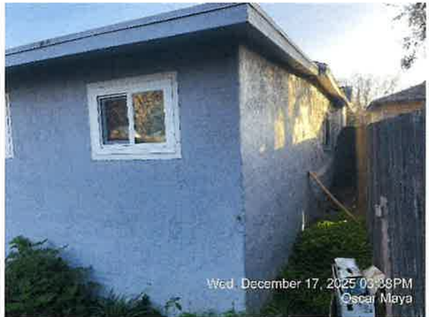
Date: 12/17/2025 03:38:45 PM Violation 2: Enclosed patio without permits.
