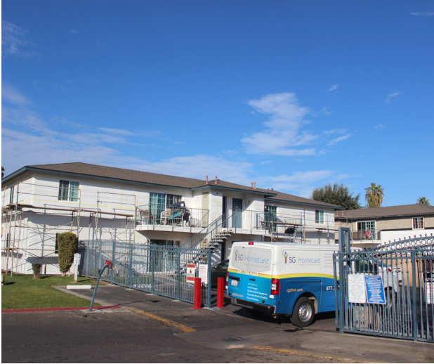
Housing in need of repair in CSE Fresno
