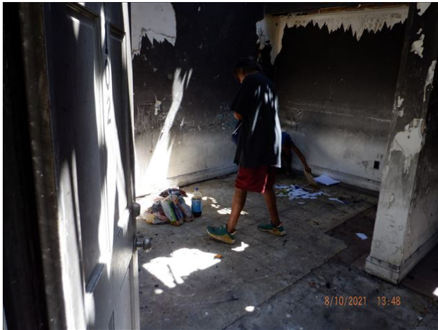
Date: 8/10/2021 1:48:10 PM Transients inside north unit. TDS
