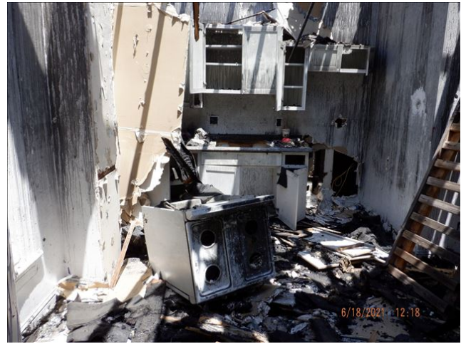
Date: 6/18/2021 12:18:11 PM Multiunit dwelling severely damaged by fire found open at multiple locations and indications of person(s) scavenging materials from what remains. TDS
