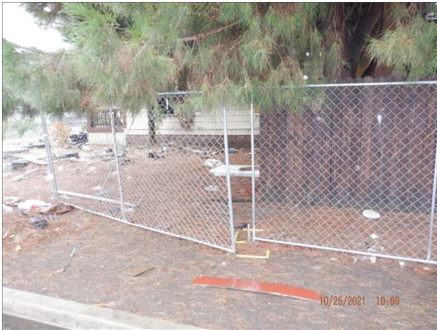
Date: 10/25/2021 10:09:53 AM Temporary fence panel left open at north elevation. TDS
