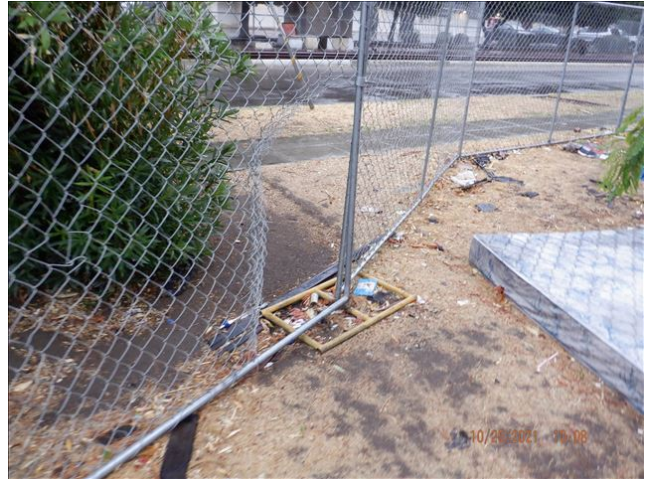
Date: 10/25/2021 10:08:22 AM Cut opening remains in temporary fence at north-east corner of property. TDS
