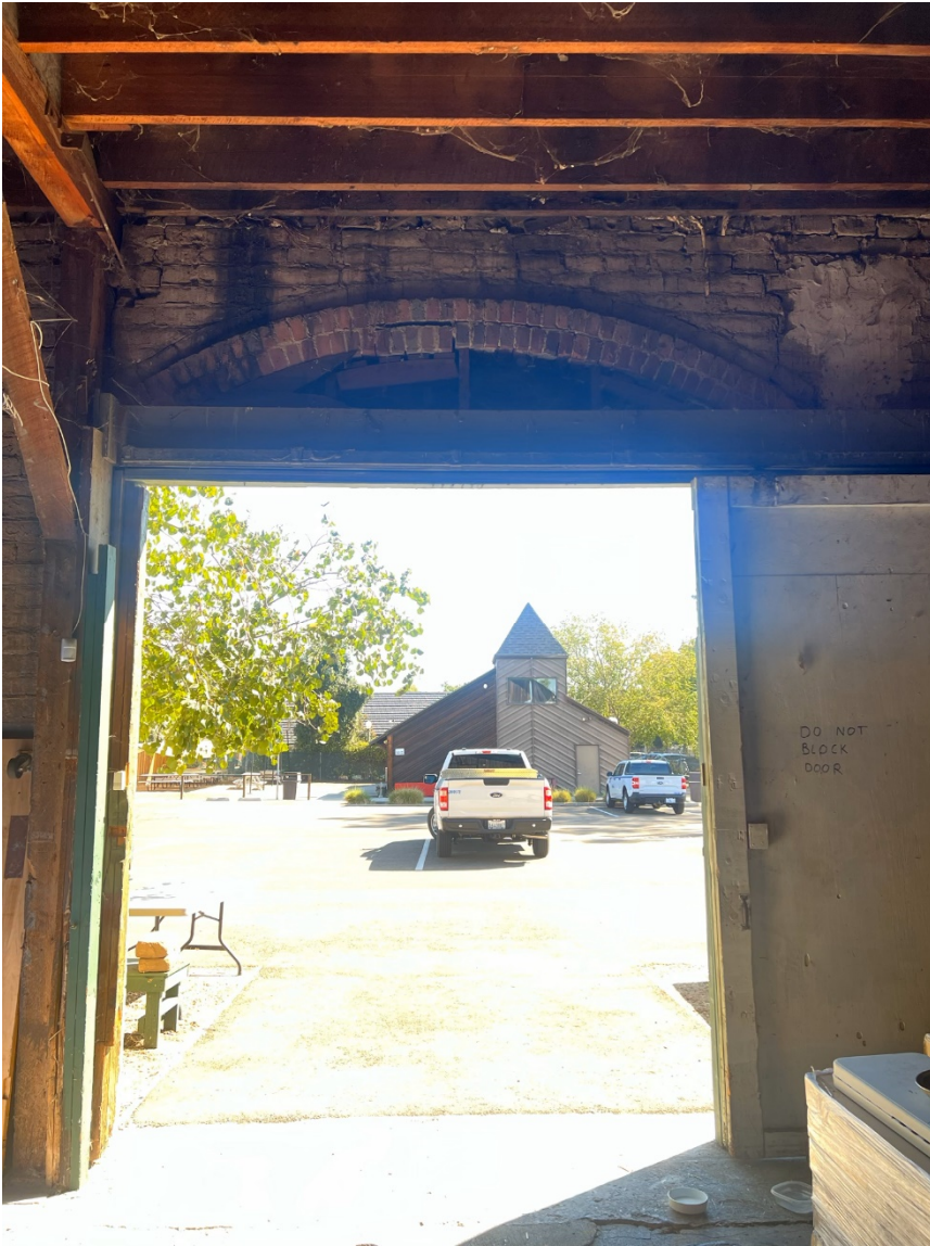
Photograph No. 5 Adobe and brick archway presenting cracks and deflection
