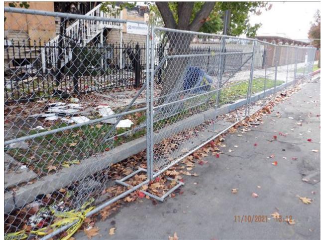
Date: 11/10/2021 1:12:04 PM Opening cut in temporary fence panel on San Joaquin side of the property. TDS
