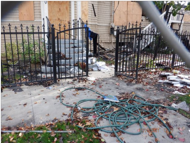
Date: 11/10/2021 1:11:58 PM San Joaquin side of property appears to have been entered within temporary fence boundary. TDS
