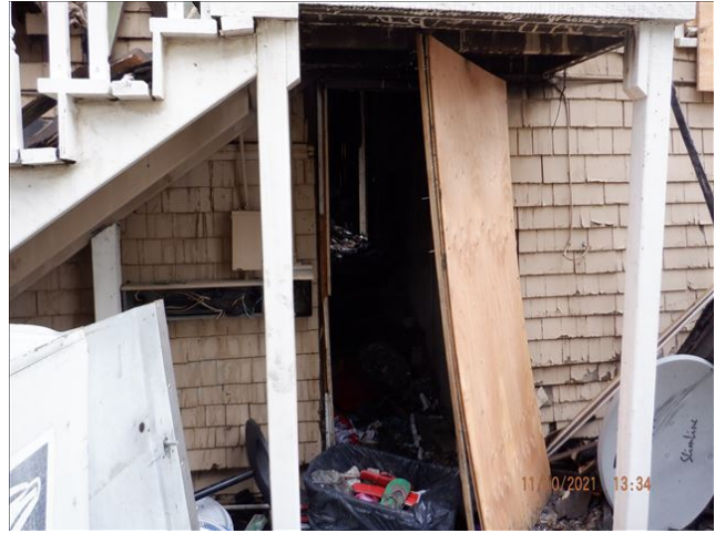
Date: 11/10/2021 1:34:32 PM Boarded entrance at north side has been forced open. TDS
