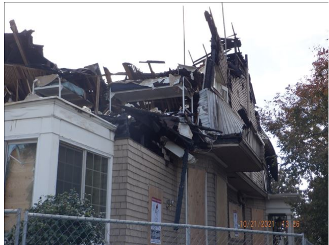
Date: 10/21/2021 1:26:33 PM Second story portion of exterior wall cantilevers out beyond first floor at north-west side of structure. TDS
