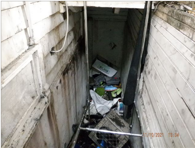
Date: 11/10/2021 1:34:59 PM Stairwell to basement inside a recently forced-open north doorway. TDS
