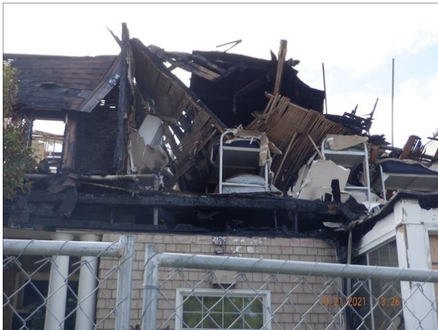
Date: 10/21/2021 1:26:13 PM Fire damage to second story at north side of property. TDS
