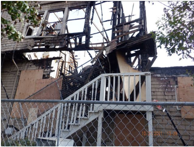
Date: 10/21/2021 1:28:56 PM Fire-damaged second story exterior wall remains largely unsupported at north side of property. TDS
