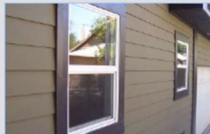
AVOID. The white window color is inconsistent with the color of the surrounding trim and cladding. White trim and perhaps a different color cladding material would result in a more consistent color palette.
