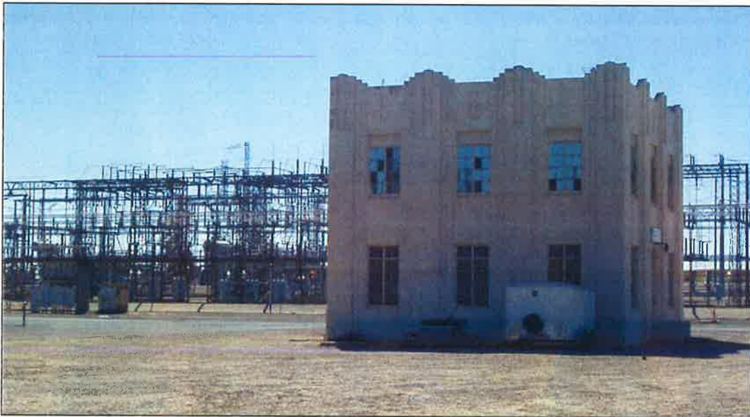
Figure 1-1 Control Building at the Herndon Substation, view to the northeast (Applied EarthWorks, August 2008).
