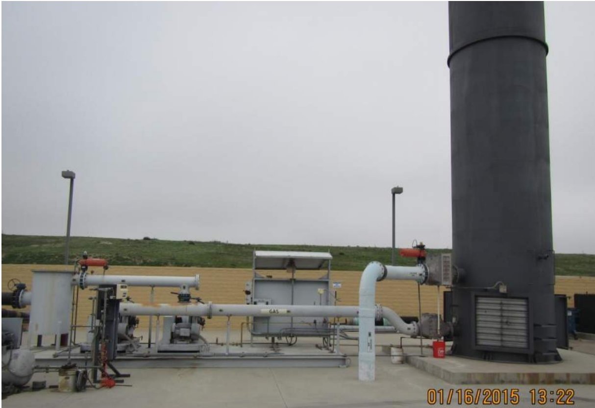
Photo 3: Landfill Gas Flare Overview
