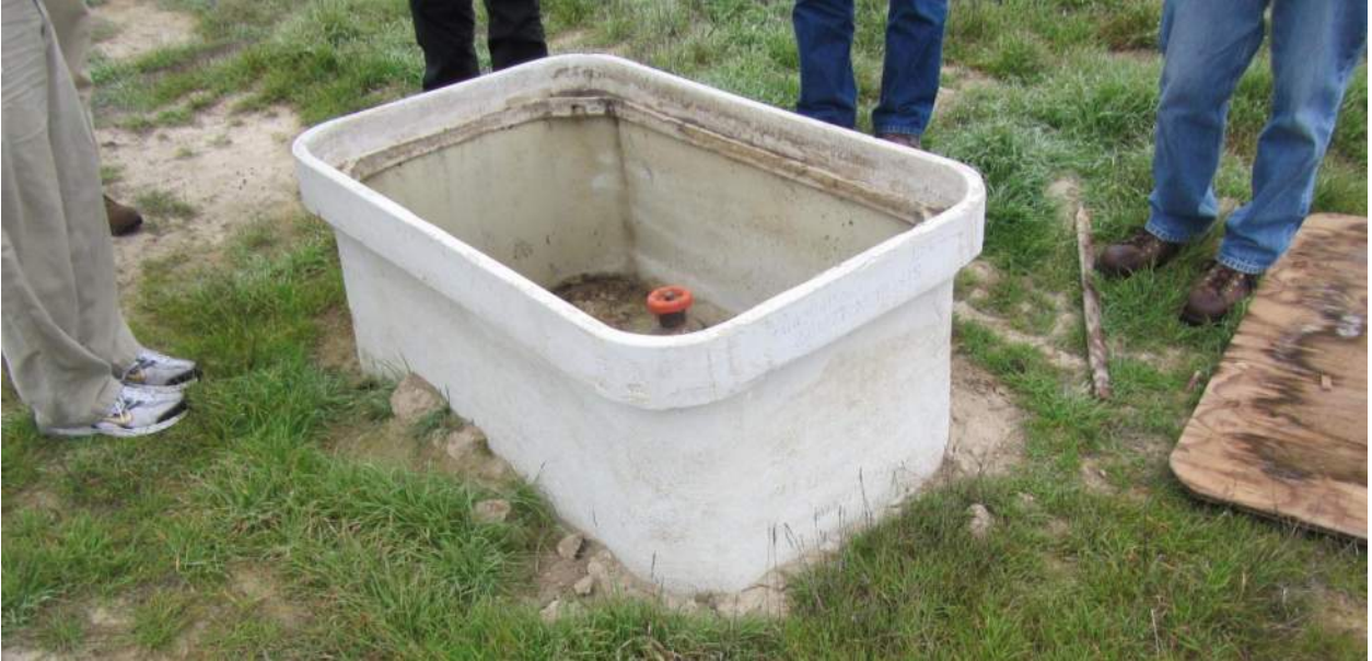
Photo 22: Gas Extraction Wellhead. Note the subsidence, as rim of well box was once at grade.
