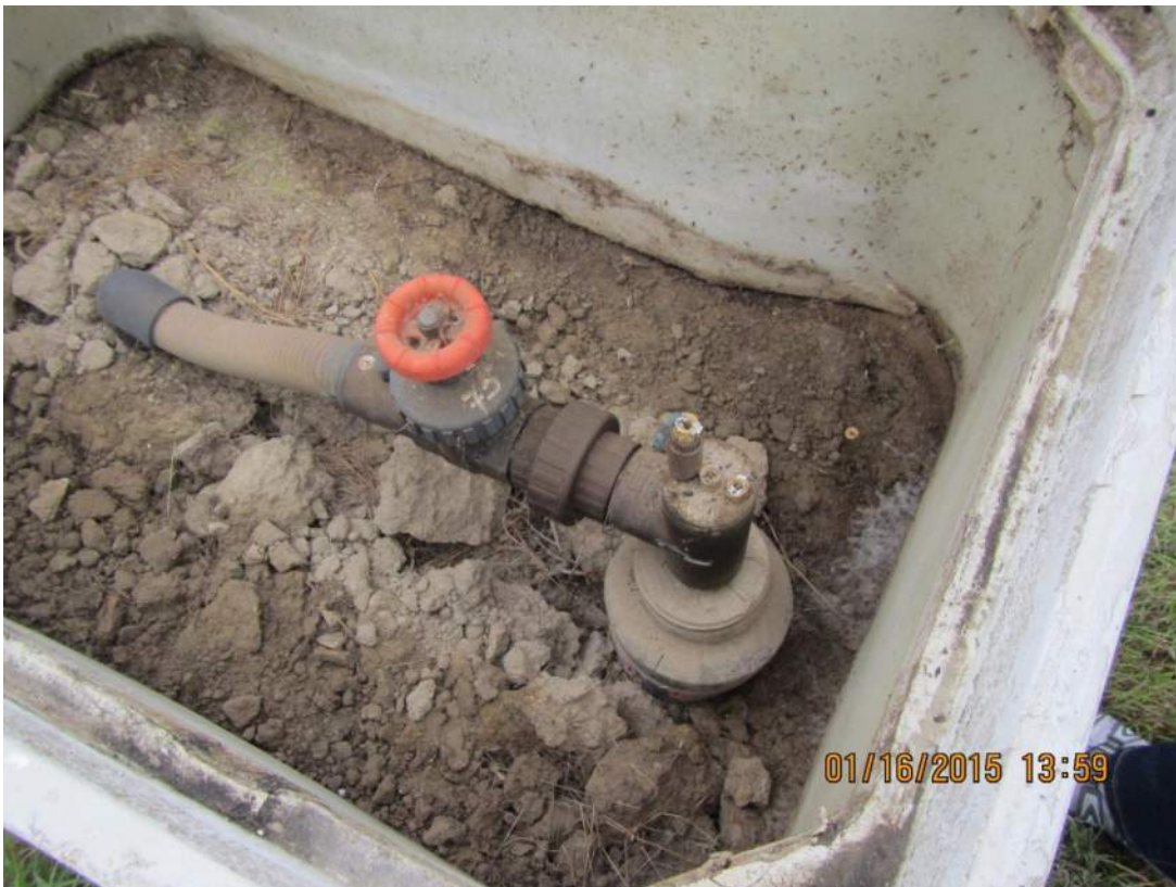
Photo 21: Gas Extraction Wellhead
