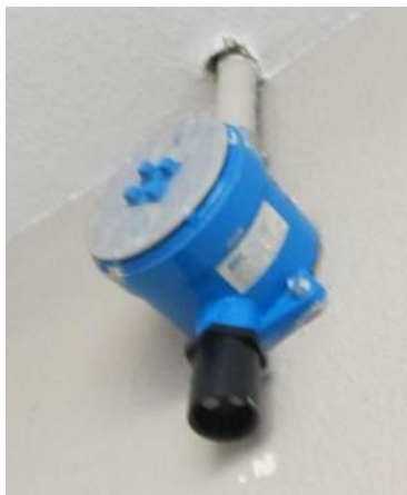
Photo 2: Gas Monitoring Device in Site Office
