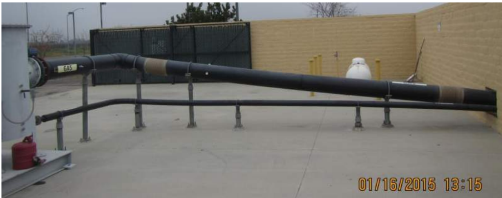
Photos 6-7: Landfill Gas Flare Detail Continued
