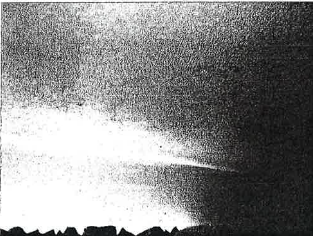
Date: 2/22/2017 8:19:26 AM CEILING REPAIR AT EAST BEDROOM WATER STAINED
