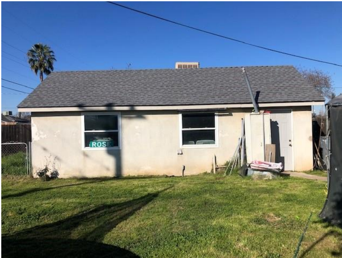
F) View looking west of the east facing façade of the detached garage. 2/28/22. Acc. #2022IMG5825
