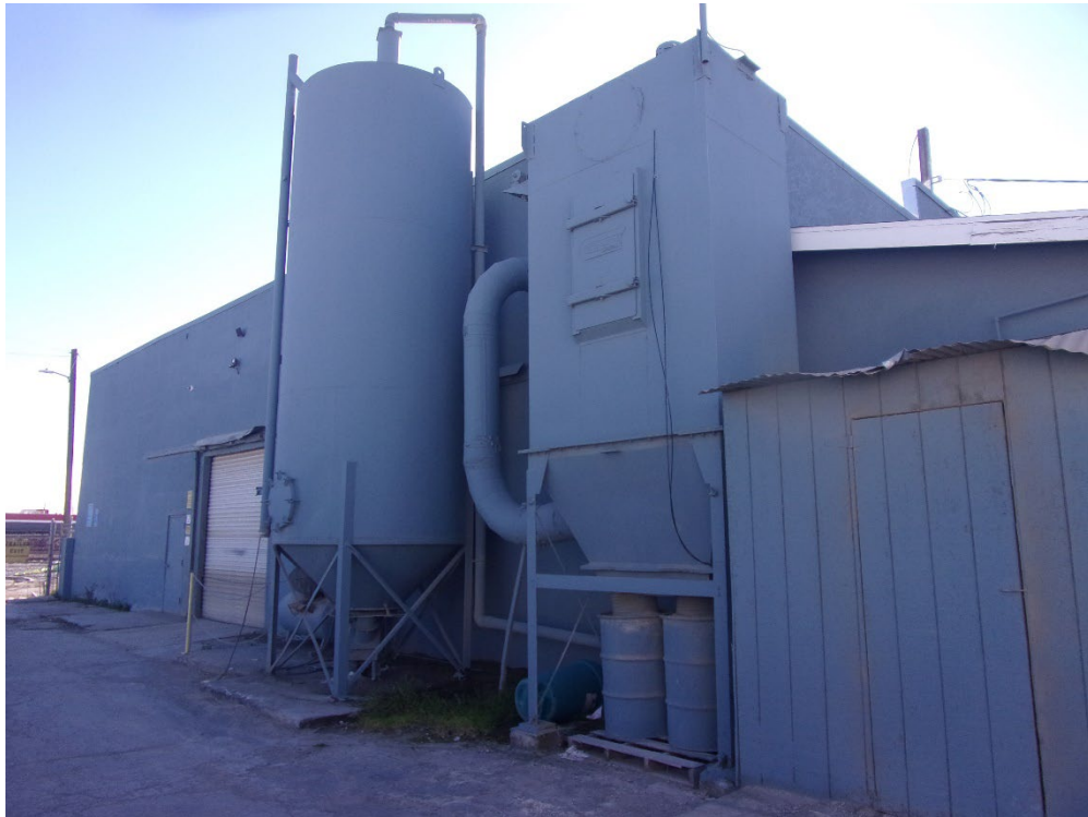
SILO & DUST COLLECTOR
