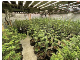
Illegal residential cultivation site that spanned 5 rooms with unpermitted electrical
