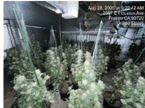
Illegal residential cultivation site with unpermitted insecticide usage, chemical storage, unpermitted electrical and ducting
