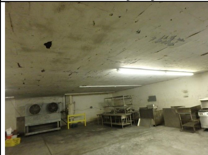
Photo 3: View of storage room 2 with ACM skimcoat
