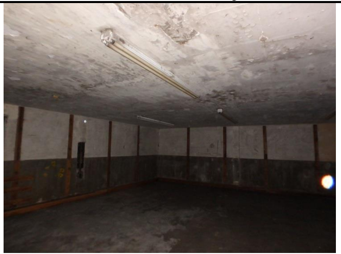
Photo 6: View of storage room 1 with ACM skim coat on the upper walls and ceiling
