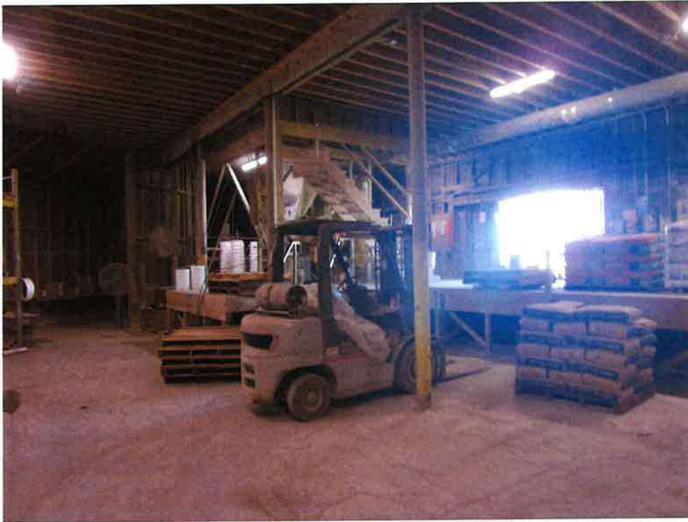
STUCCO PLANT OVERALL
