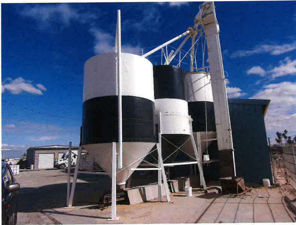
STUCCO-SAND SILOS & BUCKET ELEVATOR
