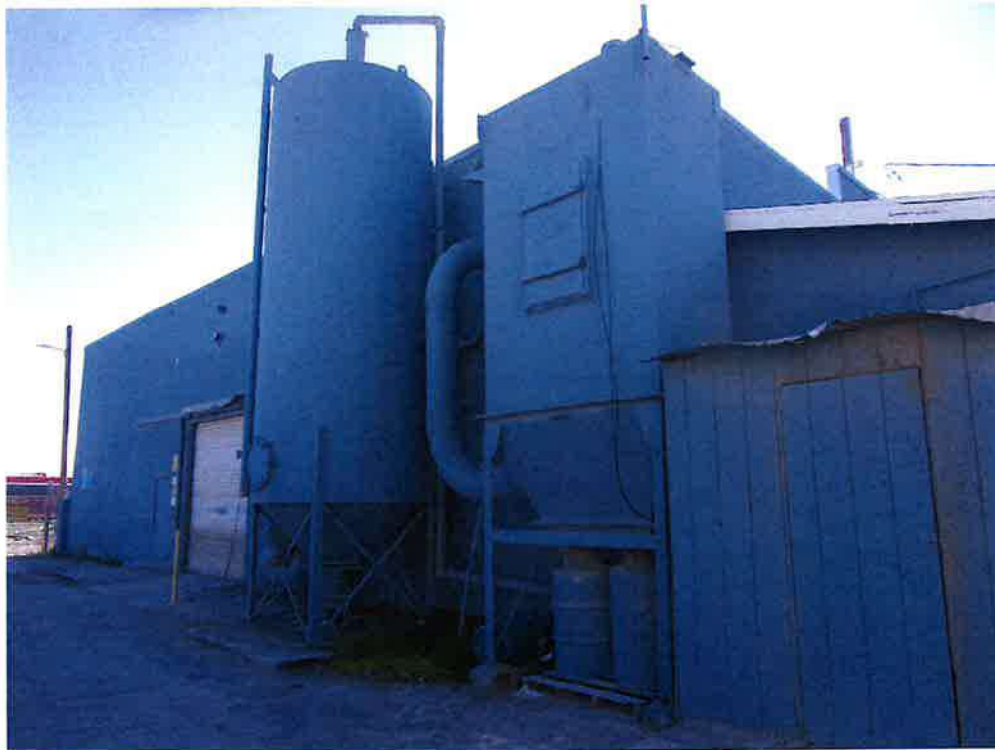
SILO & DUST COLLECTOR
