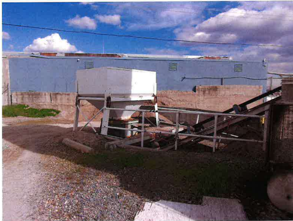
MATERIAL SCALE HOPPER & CONVEYOR
