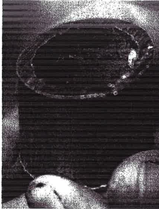
Figure 2-7. Iron-oxide accumulation on Fresno galvanized pipe.
