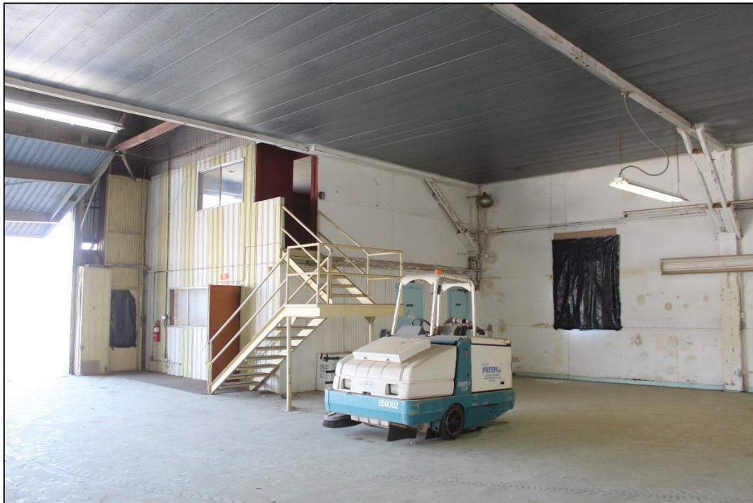
Figure 18. View of the integrated office and apartment from inside of the hangar, facing northeast (Stantec, 2025).
