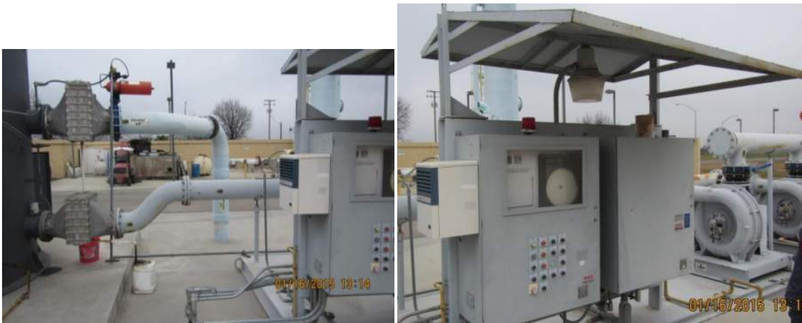
Photos 4-5: Landfill Gas Flare Detail
