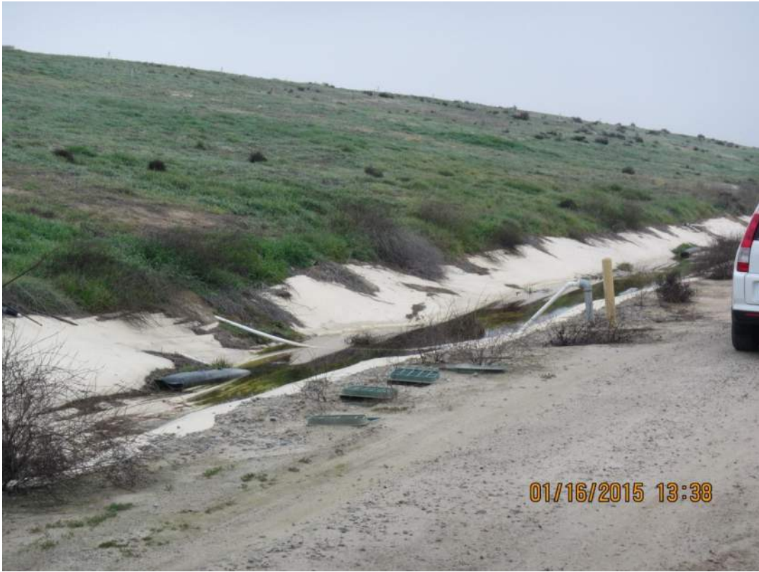
Photo 26. Surface drainage ditch on the east side of the landfill. Due to subsidence, ditch is now lined.
