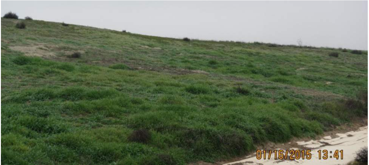
Photo 16: Subsidence on Eastern Face of Landfill
