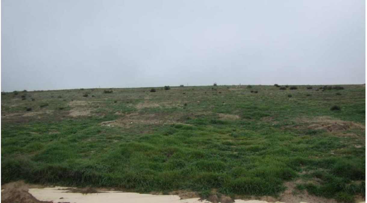
Photo 14: Subsidence on Eastern Face of Landfill
