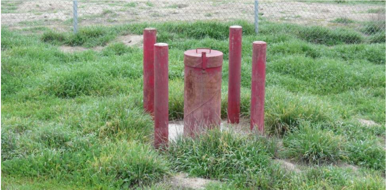
Photo 20: Perimeter Gas Well
