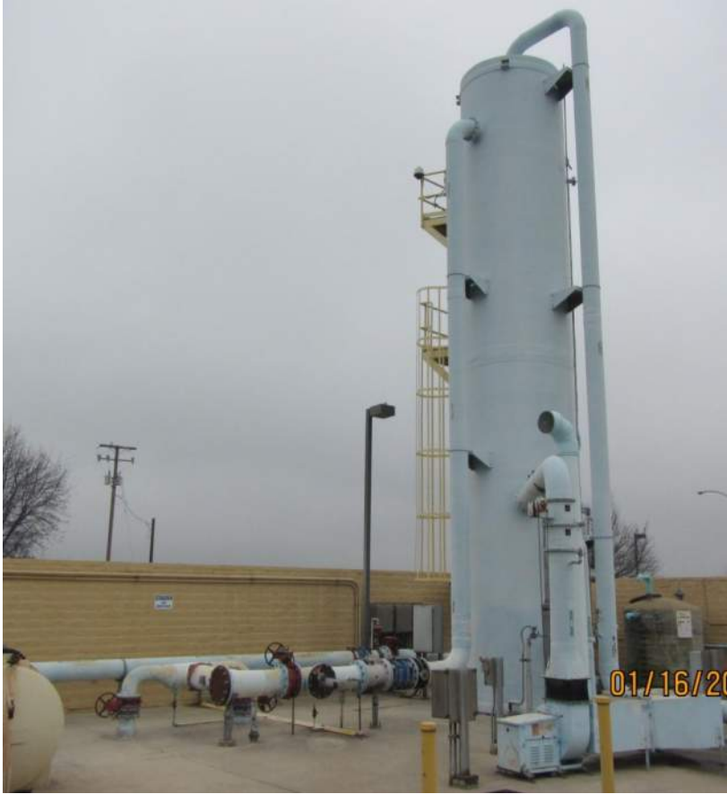
Photo 8: Packed Tower Aerator
