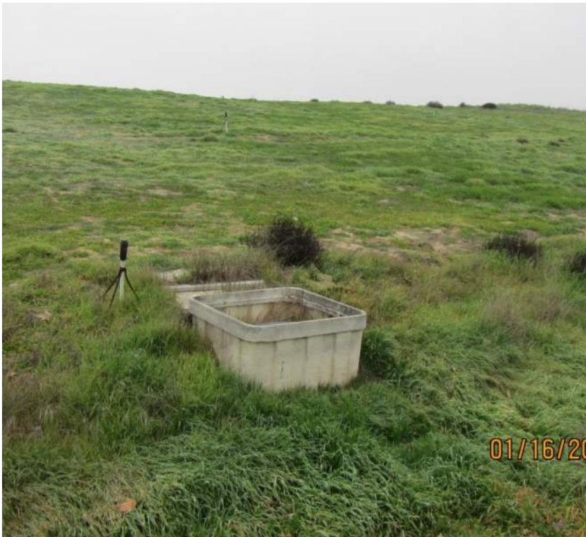
Photo 11: Landfill Gas Condensate Sump
