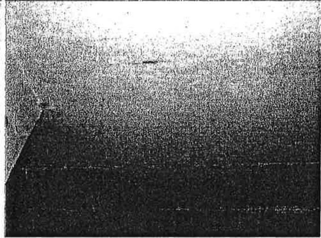
Date: 2/22/2017 8:18:19 AM CEILING REPAIR AT HALLWAY WATER STAINED.
