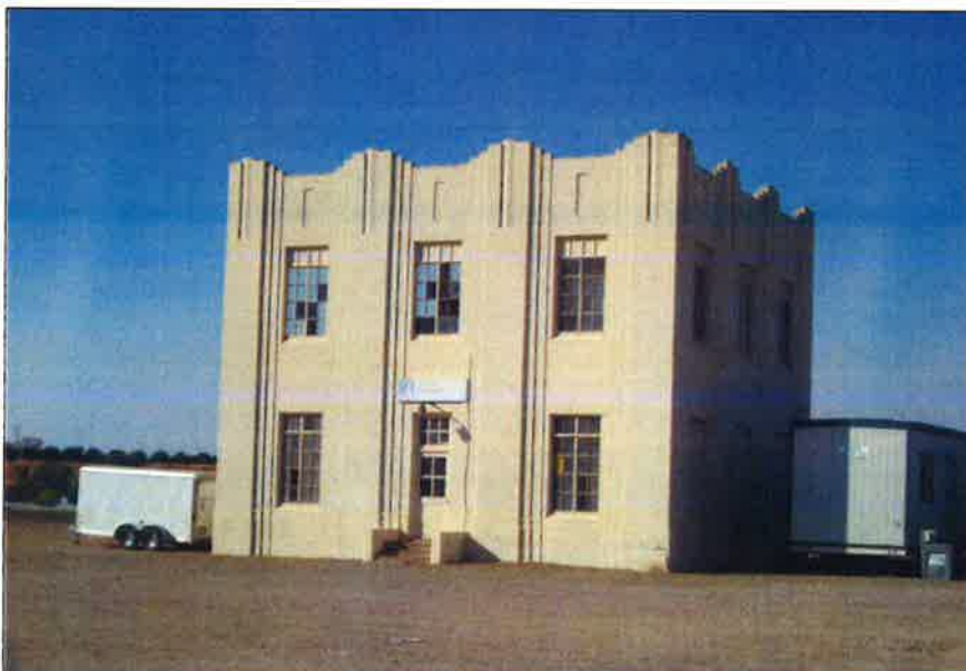
View looking northeast at west elevation of Feature I, the Control Building (August 2008).
