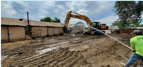
Gregory Alexander Underground Storage Tank Removal Department of General Services Role: Project Coordinator
