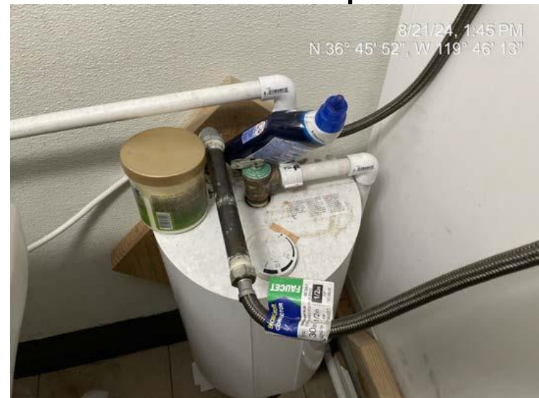
Unpermitted water heater
