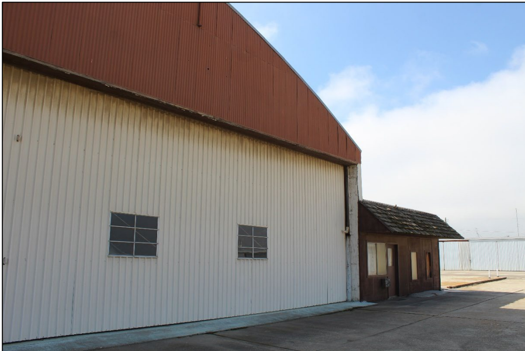
Figure 5. West end of the north façade of the hangar, facing southwest (Stantec, 2025).
