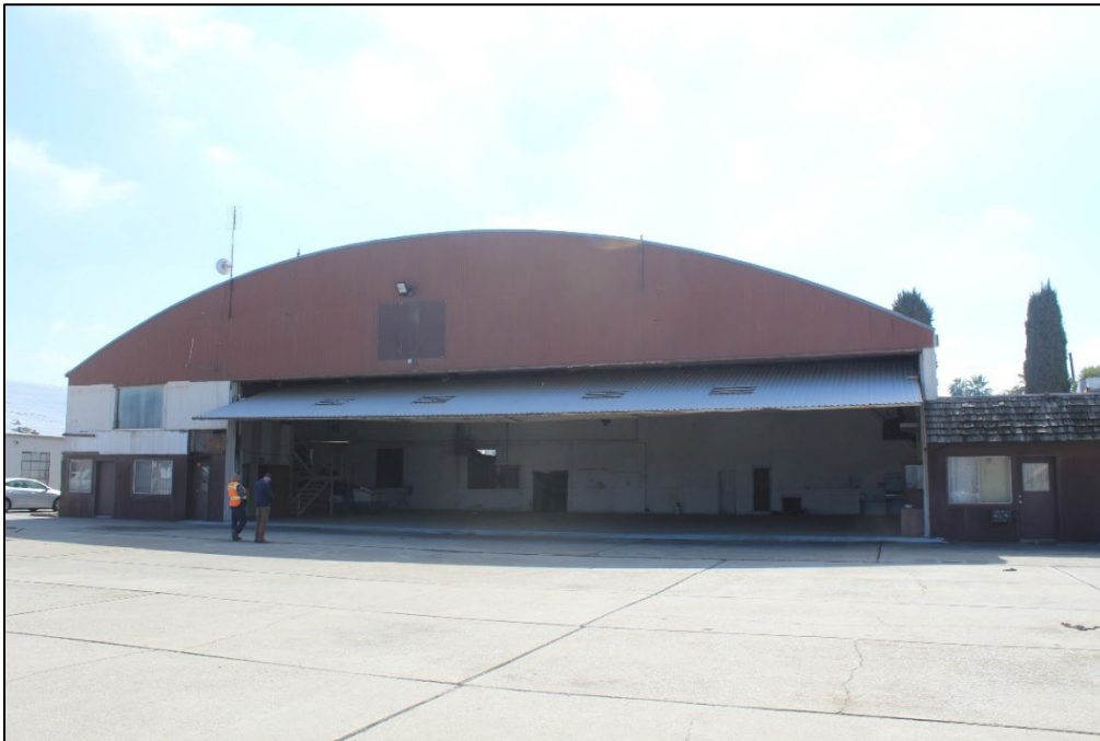
Figure 5. North façade of the hangar with open hangar door, facing south (Stantec, 2025).
