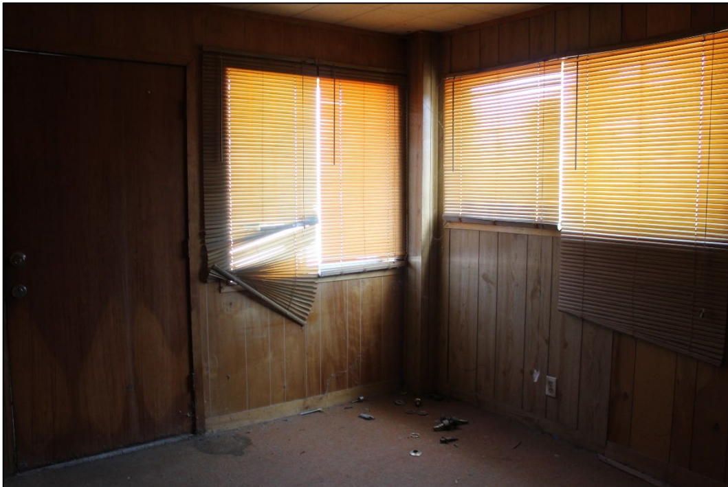
Figure 19. Interior of the first floor of the integrated office, facing northeast (Stantec, 2025).
