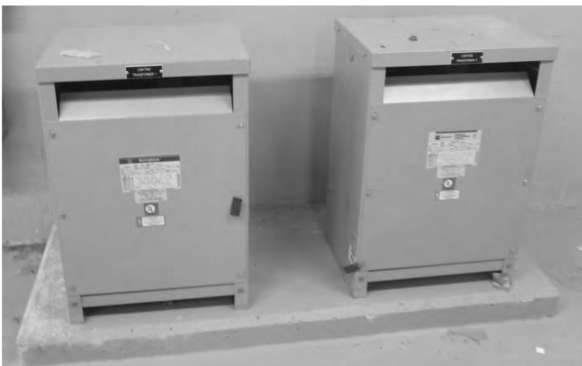
Headworks: Lighting Transformer T-1 and T-2
