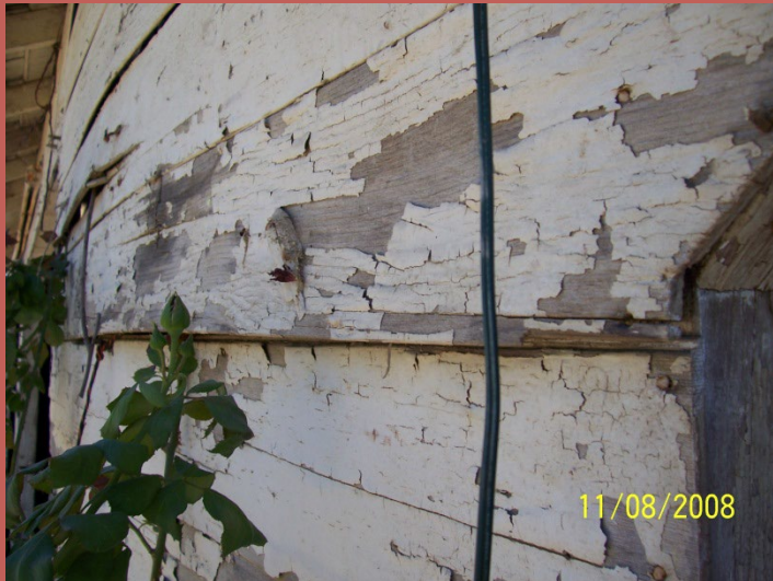
On original wood siding
