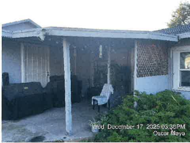
Date: 12/17/2025 03:38:27 PM Violation 1: Patio without permits.
