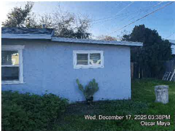
Date: 12/17/2025 03:38:31 PM Violation 2: Enclosed patio without permits.
