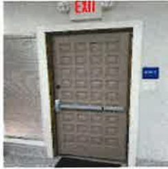
Rear exit with panic hardware
