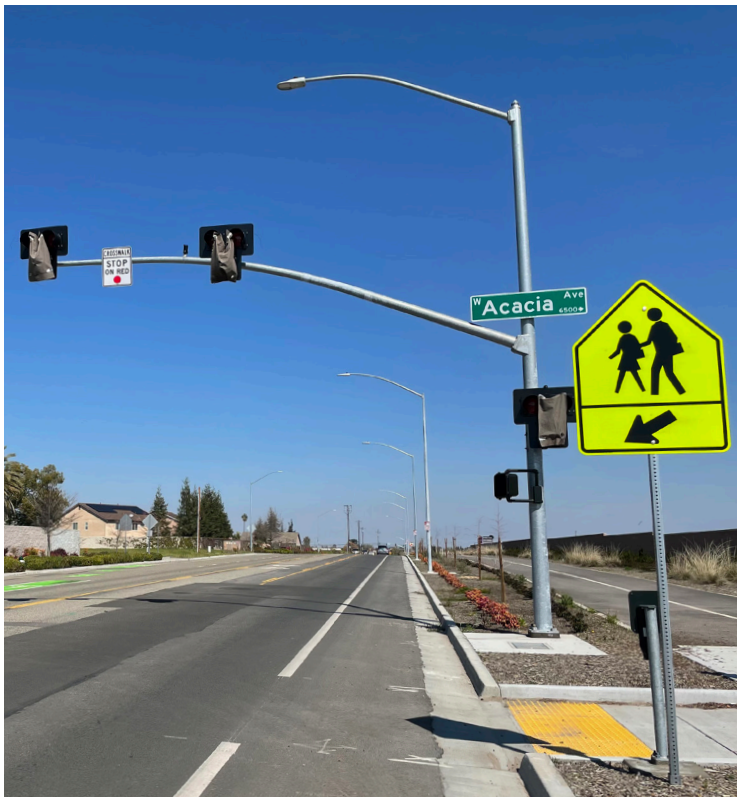
A new HAWK light being installed at the trail crossing on Bryan Avenue
