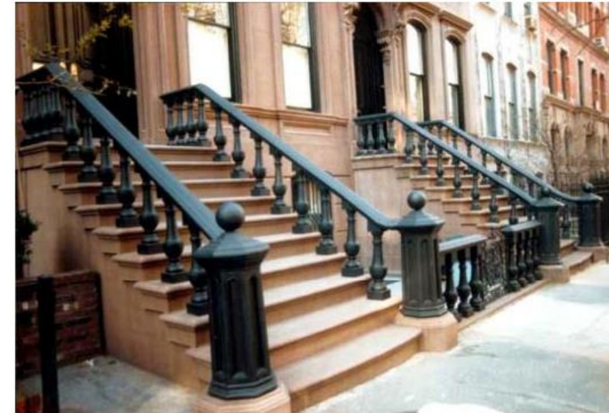
Stoops. Stoops are most appropriate for rowhouses and townhouses, but can also be used for apartment houses.
