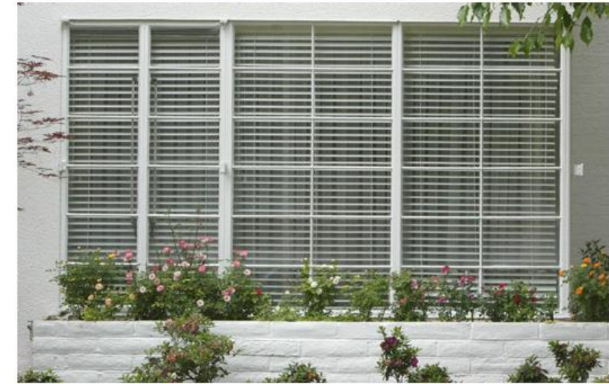
Casement Windows. If ever replaced, the pattern, size and shape of these casement style windows should be maintained.
