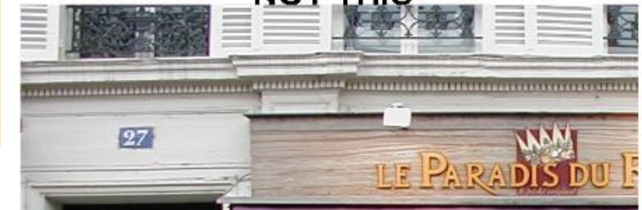
This wall sign covers up part of a pilaster and hangs over the bottom of the frieze.
